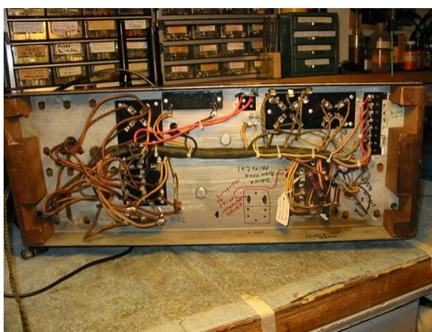
Photo #2 Underside A/PS Chassis
